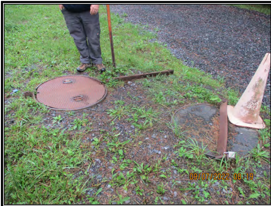
Photo No. 1 – Photo of Pressure Reducing Vault
