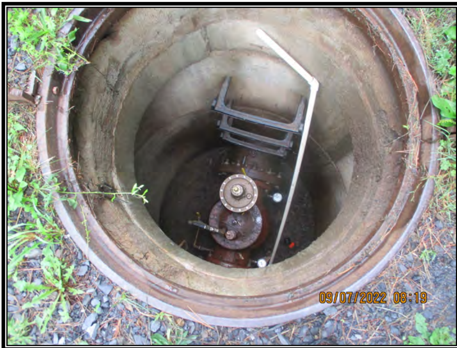
Photo No. 2 – Photo of Pressure Reducing Valve
