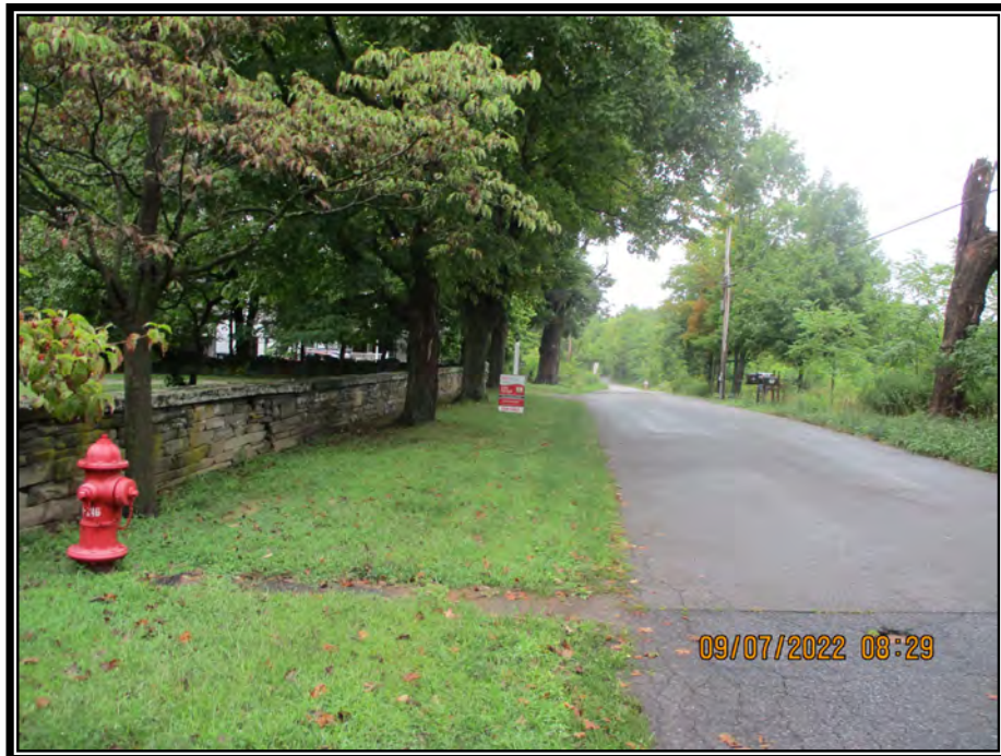
Photo No. 5 – View looking north along Huguenot Street at connection for new watermain
