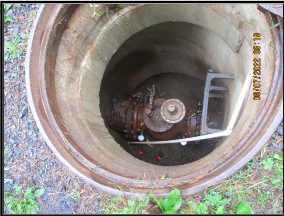
Photo No. 3 – Photo of Pressure Reducing Valve
