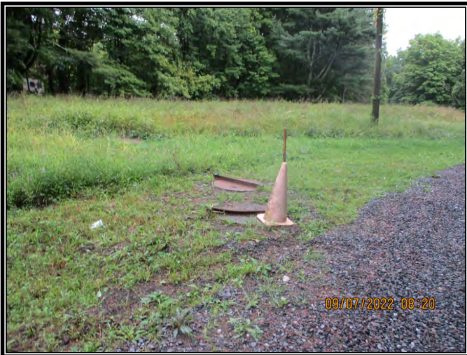
Photo No. 4 – View of Pressure Reducing Vault alongside NYC Catskill Aqueduct
